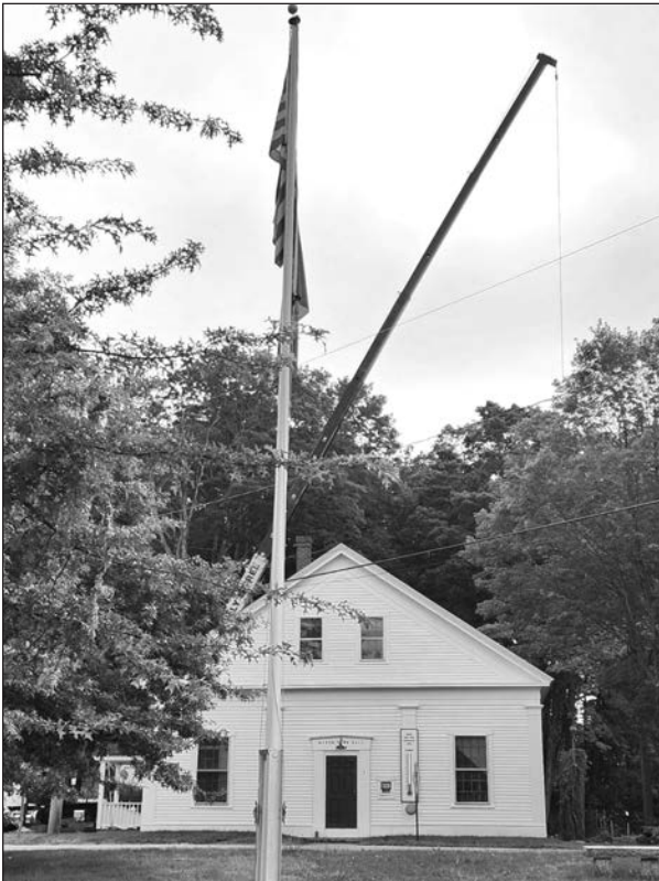
A big crane removing the large tree next to the Town Hall, which was dying and causing issues.
